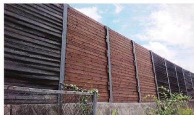
Wooden noise barrier (Nagano Prefecture) Nagano Prefecture Wood Sales Promotion Council /Wood Products Wooden noise barrier developed for the promotion of use in karamatsu (Japanese larch) of Nagano Prefecture.
